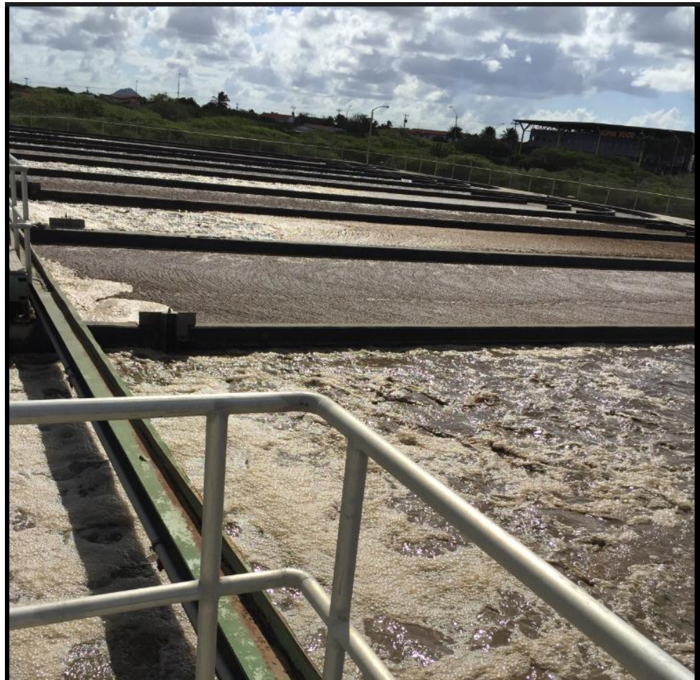
Figure 7: Aeration system of RWZI Bubali.
